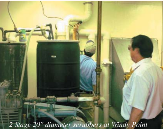
2 Stage 20" diameter scrubbers at Windy Point
