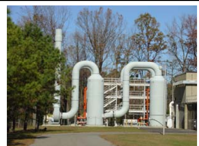
Two stage H 2 S odor control scrubbing system.
