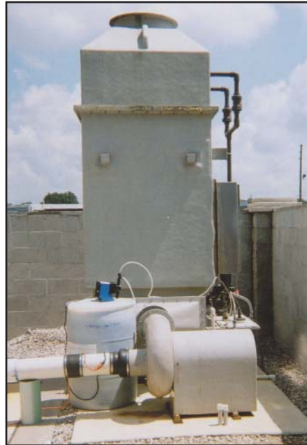
Apopka, FL Biotrickling Odor Control System
