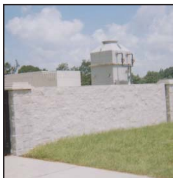
Biotrickling Odor Control System Bradshaw Road Lift Station
