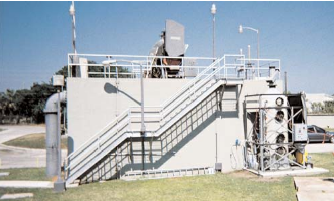
Mt. Dora WWTP Biotrickling Filter using HD Q-PAC®
