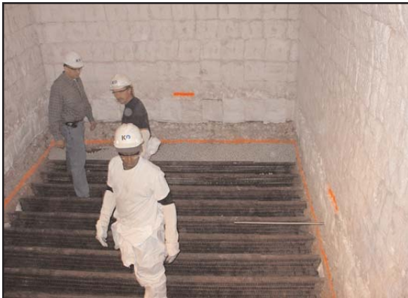
25-mm ceramic balls installed according to wall markings indicating proper level of balls and MLM®
