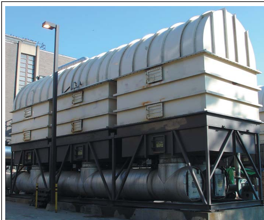
Three Canister Regenerative Thermal Oxidizer Upper Blackstone WWTP, Worcester MA Retrofitted to MLM® Heat Recovery Media October 2004
